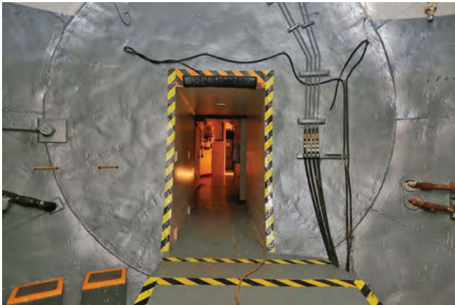
A tunnel allows access to an underground bunker housing the launch control centre
